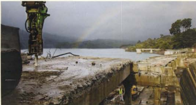
San Mateo County has completed demolition of Skyline Bridge over the Lower Crystal Springs Dam. This work clears the way for upgrades to both the Dam and the CSSA transmission system.
