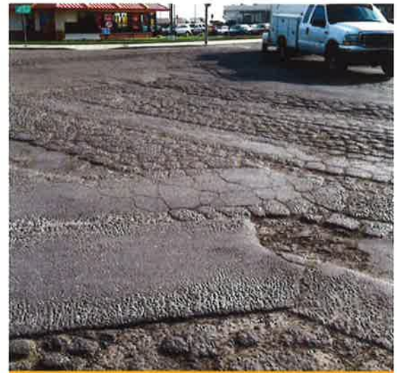
Example of worn asphalt ready for replacement along Howard Road in Westley, CA.
