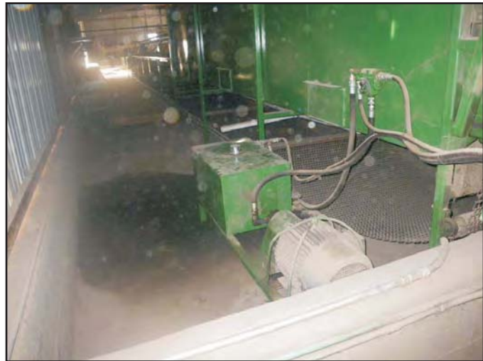
Photo 11: Hydraulic oil leak at packing machinery.
