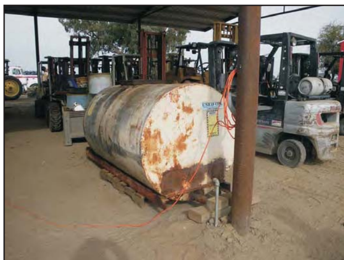
Photo 15: Waste oil tank in pole barn.
