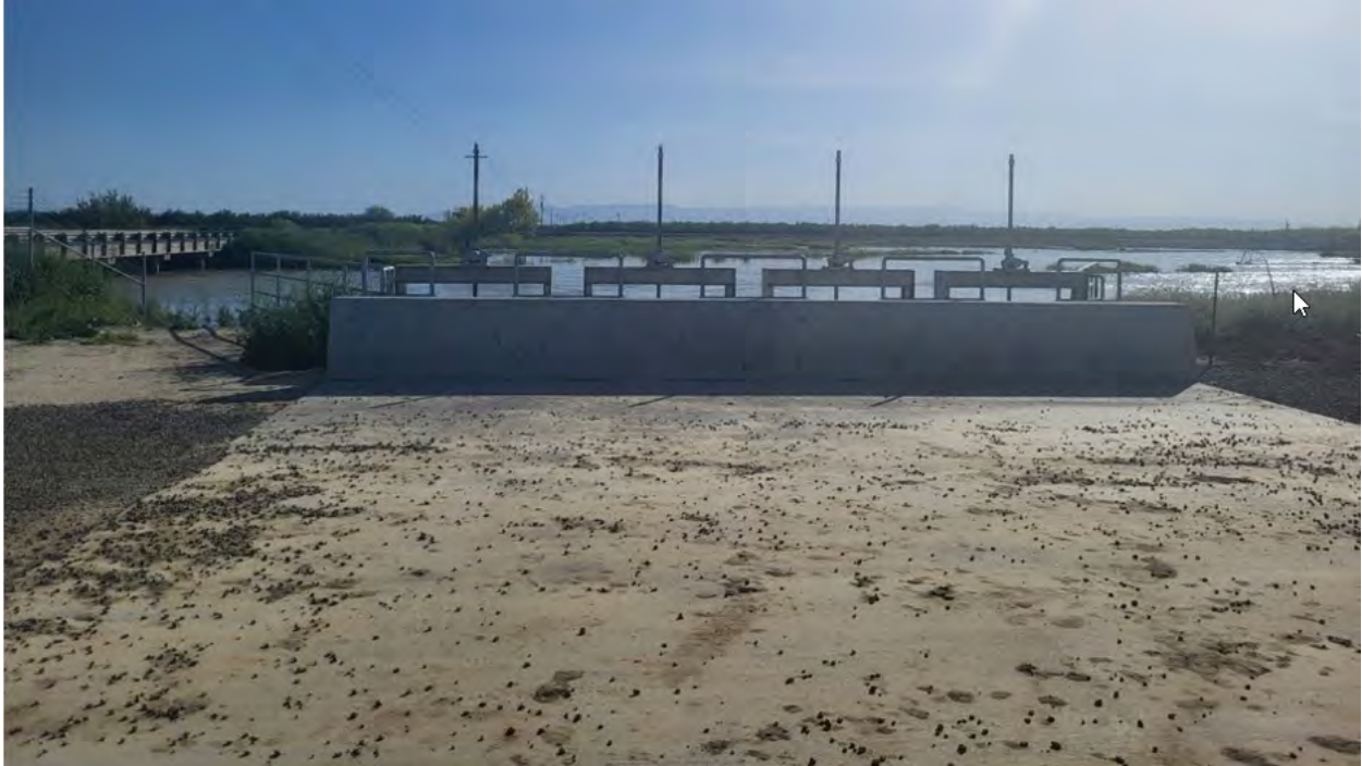
Four turnout gates on the Kings River diverting water into the Terranova Ranch canal system.
