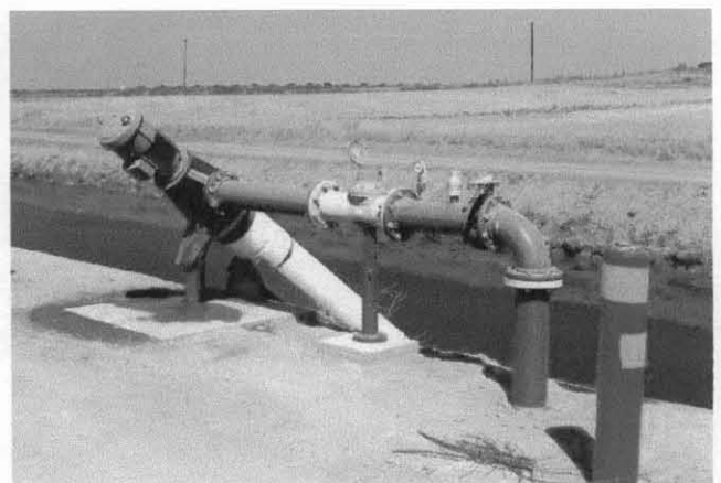
Pump in TID Highline Canal
